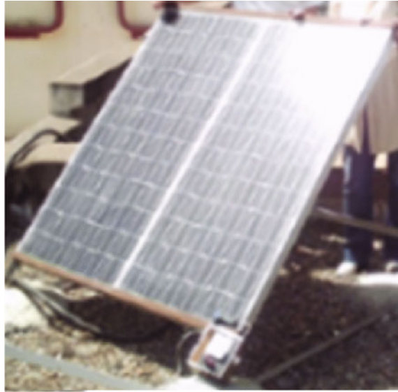
Fig. 2.10 Example of PV array structure
